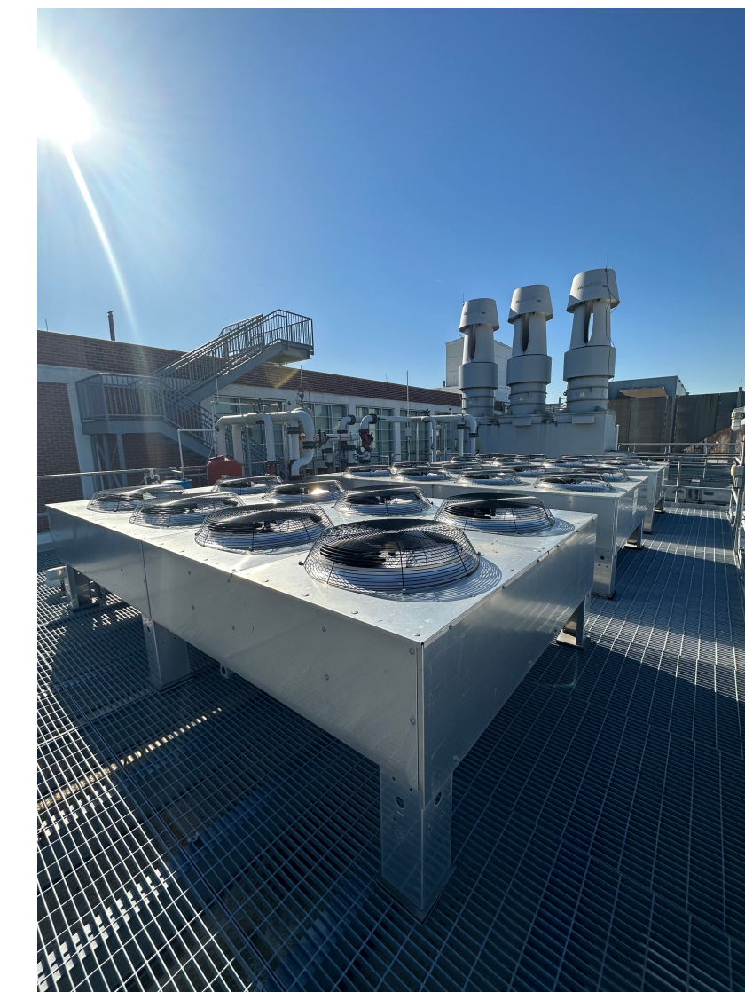
Figure 5: Center roof cooling equipment
